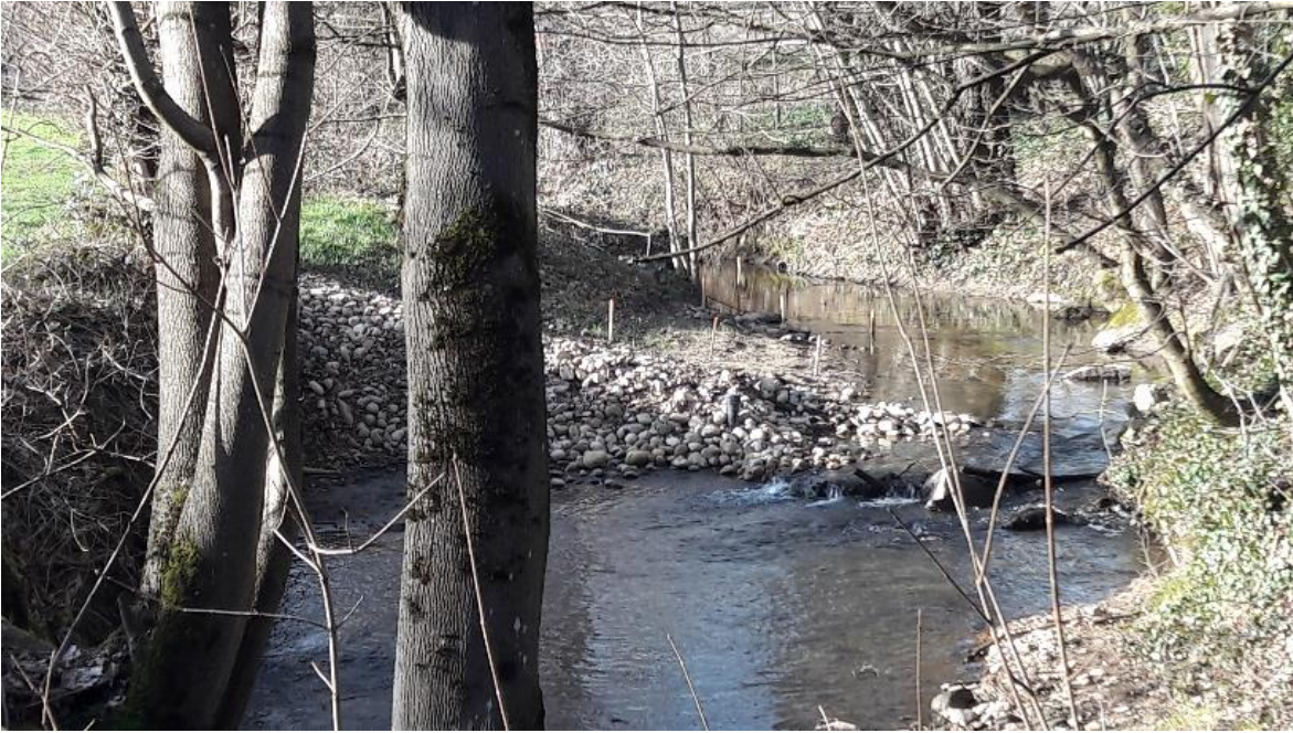
Figure 4. Porous Ramp System in the Ratier River - Equipped with wooden sticks upstream to monitor the formation of the sand biofilter. (Construction: Green Style, INRAE Designer, Owner: SAGYRC - Syndicat fluvial France).
