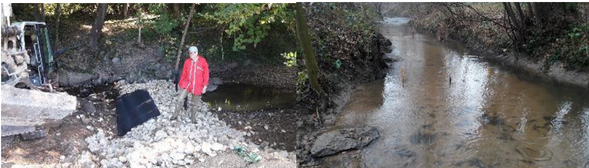
Figures 2 and 3. Implementation phases of a porous ramp: left- stony ramp shaping across the Ratier little river, right – sand accumulation acting as biofilter upstream the porous ramp after 8 months of functioning.
