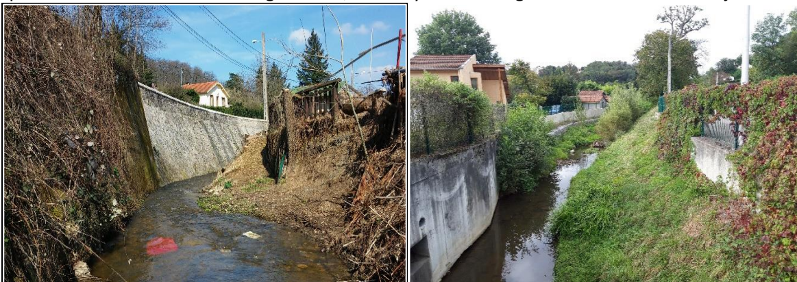
Figure 2.2. Example of stone and concrete walls to protect a road and houses against flooding. View taken upstream of the ATENAS demonstration site, near the city of Lyon. The result is a deepened and straightened riverbed.
