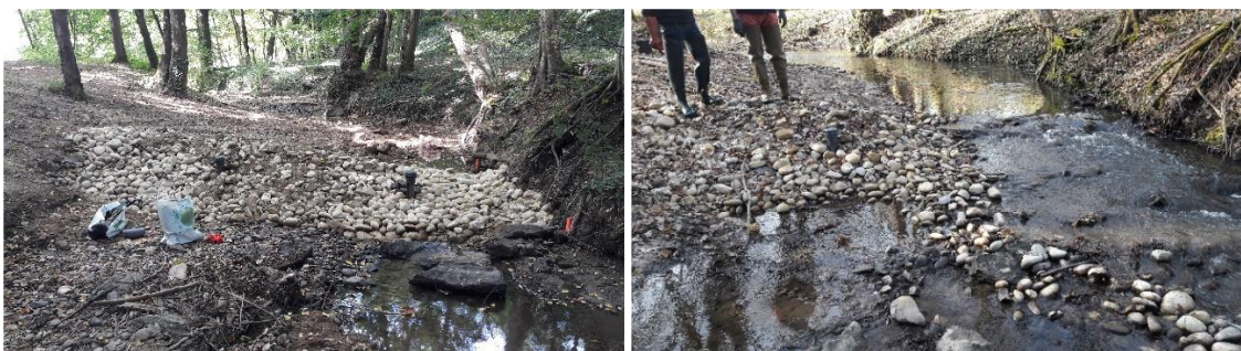
Figure 2.11: Example of erosion of the nose of porous ramp number 2 (left = before; right = after).
