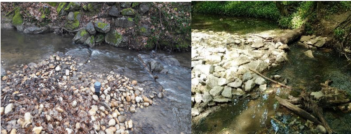
Figure 2.7. Reconstruction of the porous barrier nose. Condition after major flooding (left) and after more resistant reconstruction (right).
