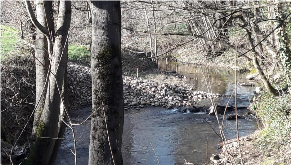
Figure 11. Porous Ramp System in the Ratier River - Equipped with wooden sticks upstream to monitor the formation of the sand biofilter. (Construction: Green Style, INRAE Designer, Owner: SAGYRC - Syndicate fluvial France).
