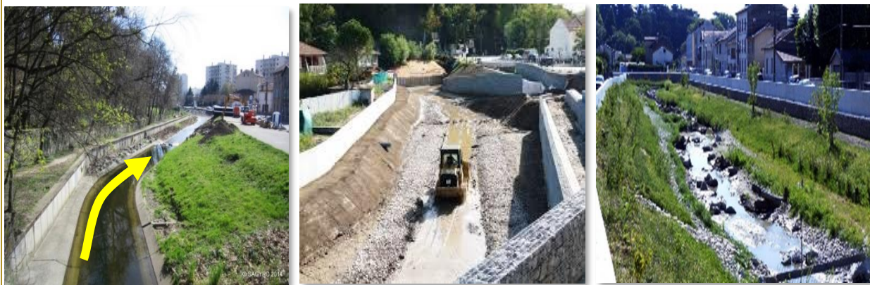
Figure 10. Before restoration (4 m wide concrete channel)-> during work (concrete bed removed and river width widened to 20 m with solid fixing in the ground to withstand a 30-year flood)-> after one year of operation (footpath visible next to gabion line).
