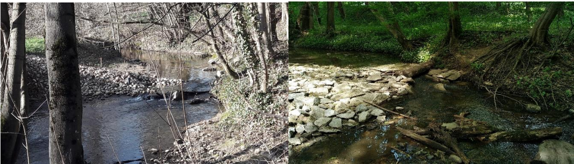
Figure 21. Eroded (left) and repaired (right) porous barrier.
