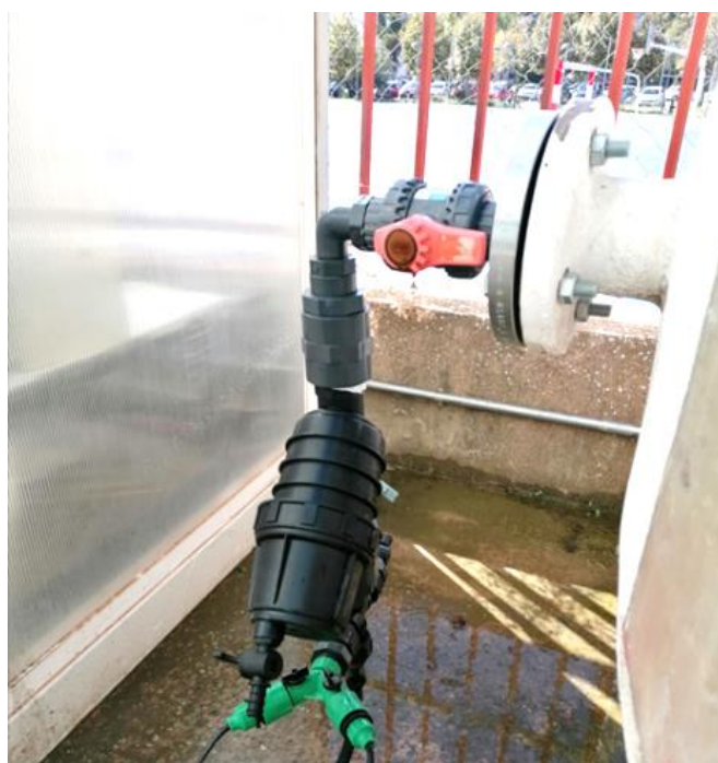
Figure 3: Filter installed at the outlet of the feed tank to the SERPIC treatment plant.
