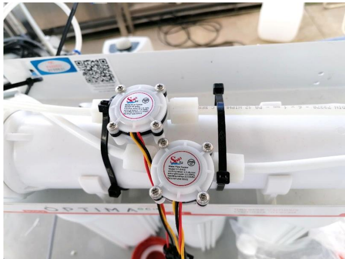
Figure 4: Flow meters in the concentrate and permeate flow.
